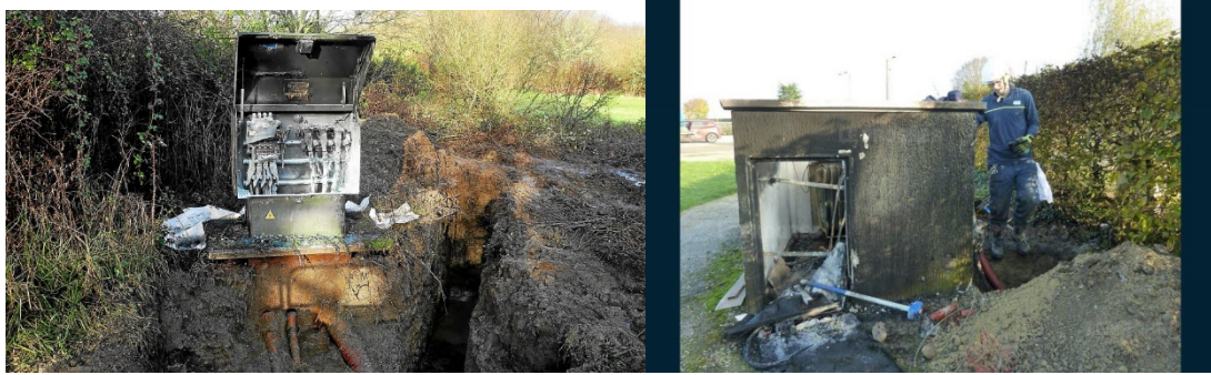
Figure 2.3 After Transformer Explosion, Soil Should Be Checked for any Possible Soil Pollution
