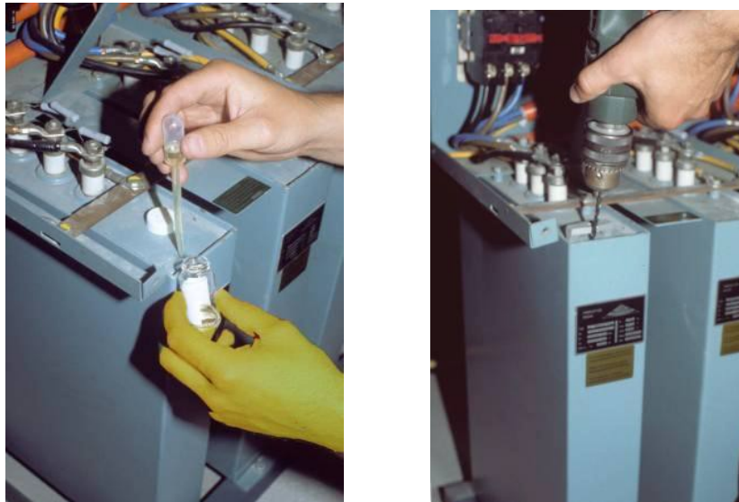
Figure 3.11 Identification of PCB Containing Capacitors
