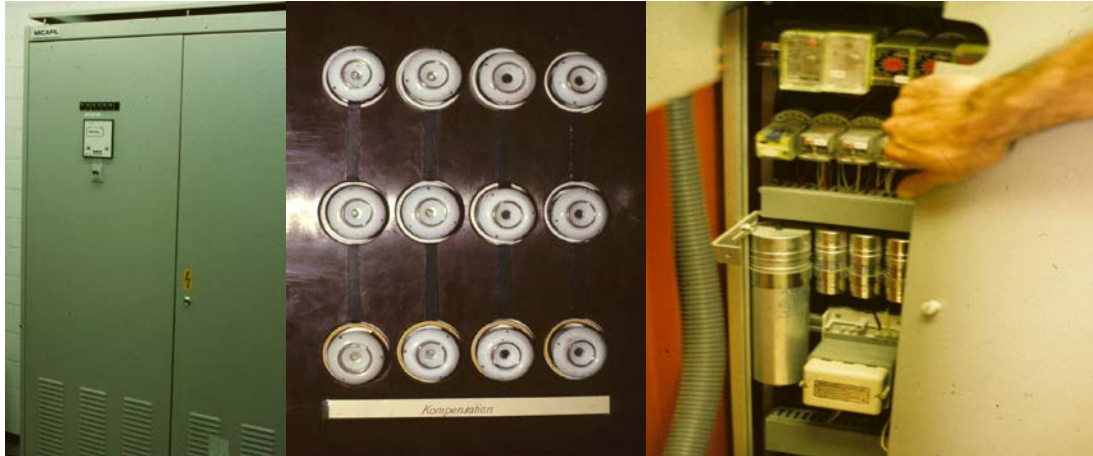
Figure 3.10 Different Types of Condensers and Capacitors in Storage or Use
