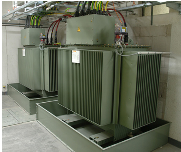
Figure 3.12 Retaining storage pan for PCB-containing transformers
