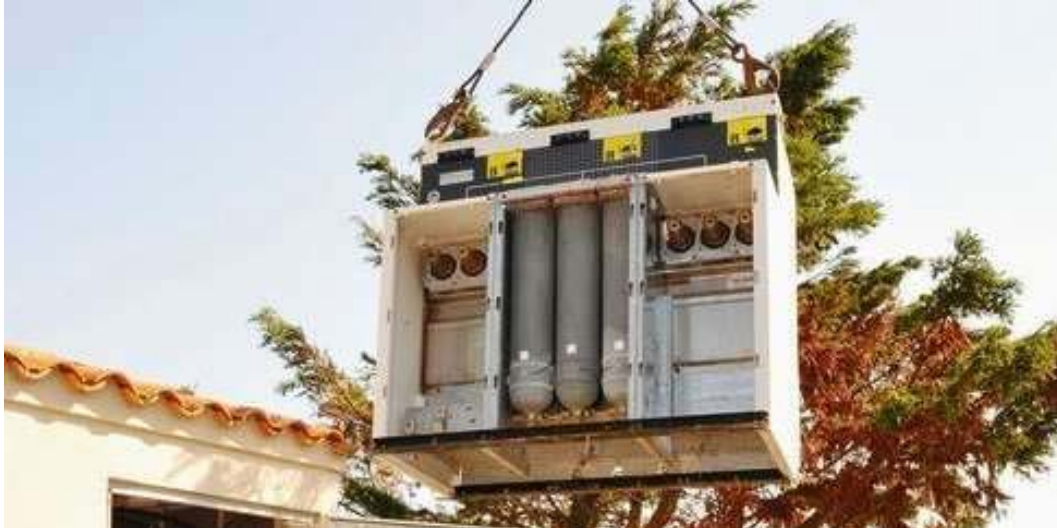
Figure 3.8 Corroded Transformer Exposed to Salt (French West Coast)
