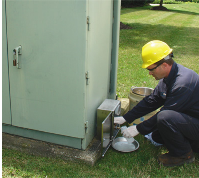
Figure 2.7 Sampling from the Valve of the Transformer
