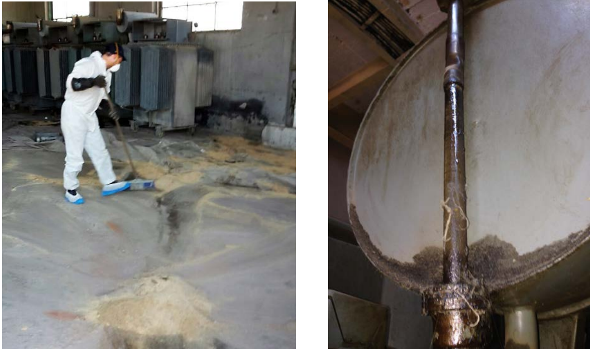
Figure 3.6 Leakage on an Old Transformer (Manufacture Year: 1975)
