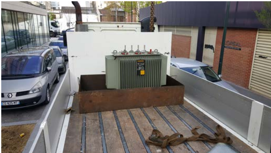
Figure 5.7 Truck Platform Double with a Liquid Retention Steel Tank
